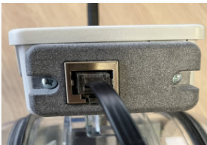
3/ Check the cable is well connected then do the same with the other e-VAV
